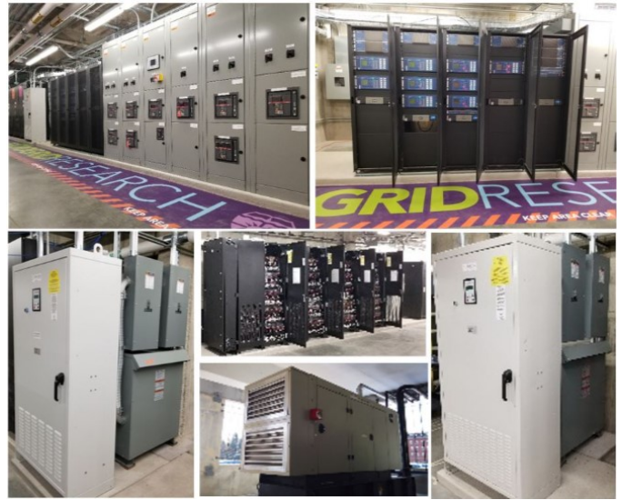
Fig. 2. Legacy power devices at the CMR Microgrid: SEL relays, PV array inverter, Battery inverter, and a Diesel Generator. Cited from Fig. 3. [10]
