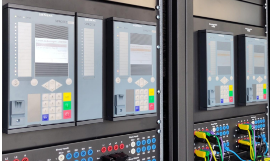
Fig. 1. Hardware setup of the implemented IEDs.
